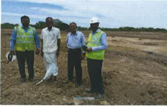
Village pond deepening activity at Thamaraiikulam being inspected by Civil Engineering team from DCBL-Ariyalur
