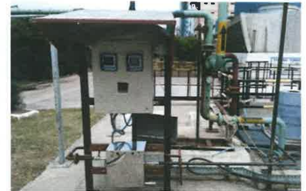
Online Monitoring at ETP
