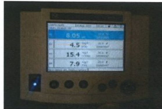
Online Monitoring at STP
