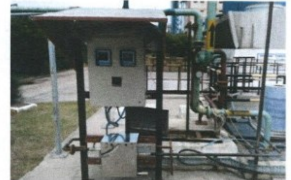
Online Monitoring at ETP
