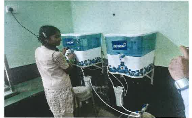
RO Plant 25 LPH at Edayathankudi Govt school
