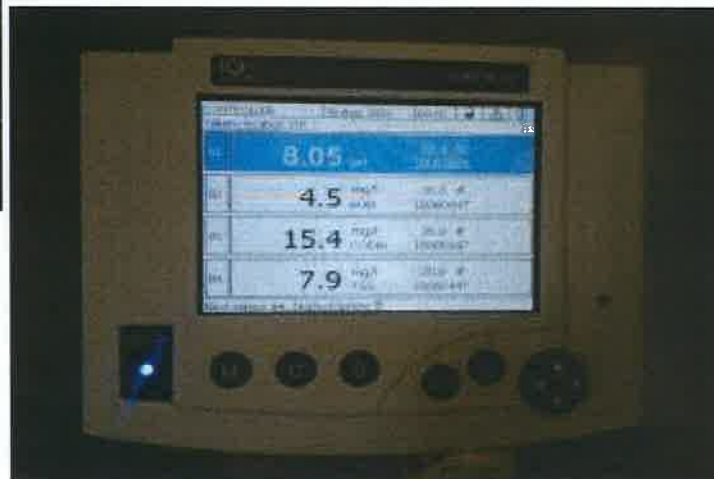
Online Effluent monitoring system at STP
