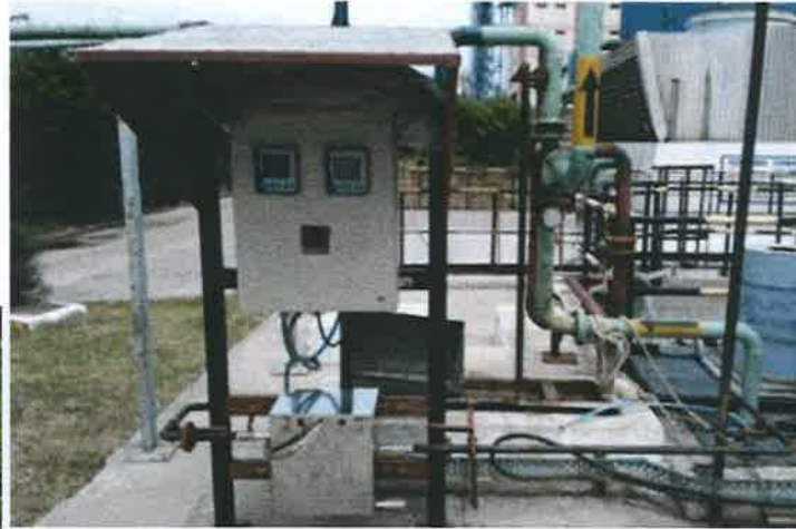
Online Effluent monitoring system at ETP
