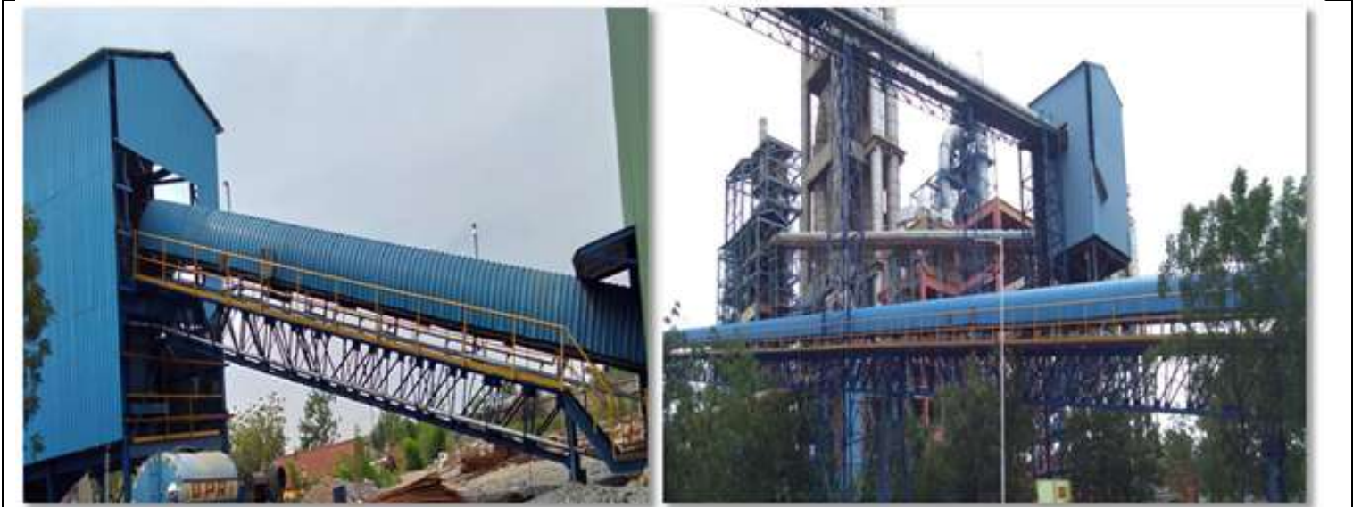
Covered Conveyor Belts
