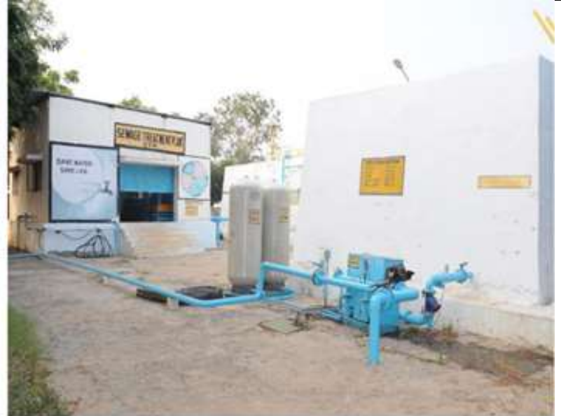
Sewage Treatment Plant
