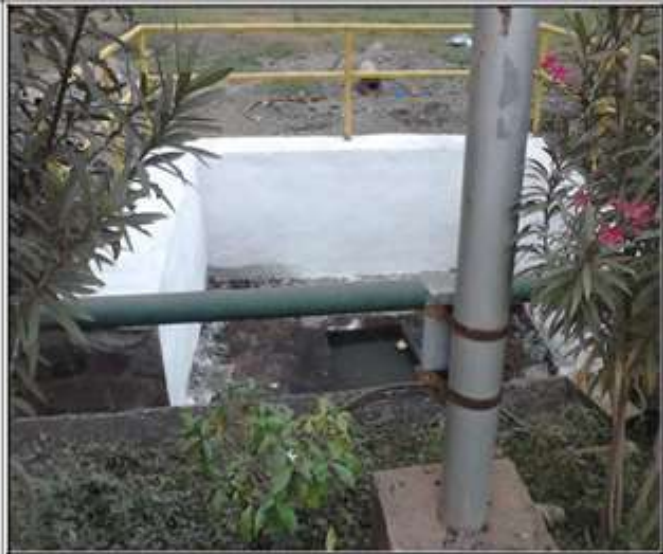
Rain Water Harvesting
