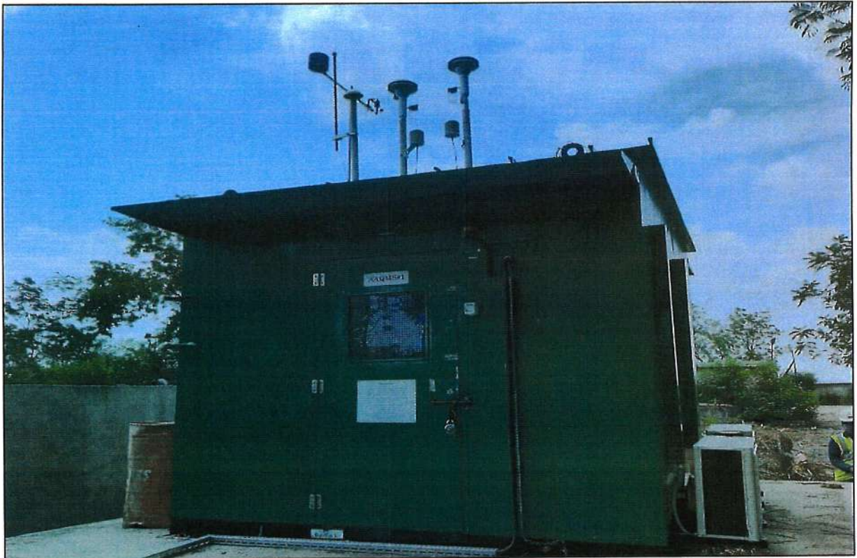
CAAQMS -01 installed at Plant Main Gate
