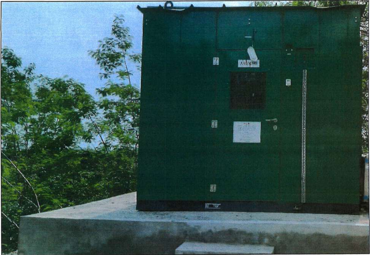
CAAQMS -03 Installed at Crusher Area (Mines)
