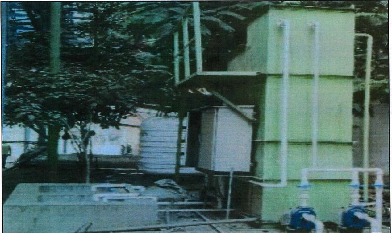
Sewage Treatment Plant Installed at Packing Plant Area
