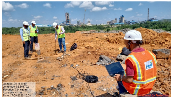
Fig. 21. Lowering of piezometer at the borehole#1 with a depth of 171bgl in the location 92°21' 42.45"E - 25°10'58.65"N at the Umsoo Mootang mine in September, 2023.
