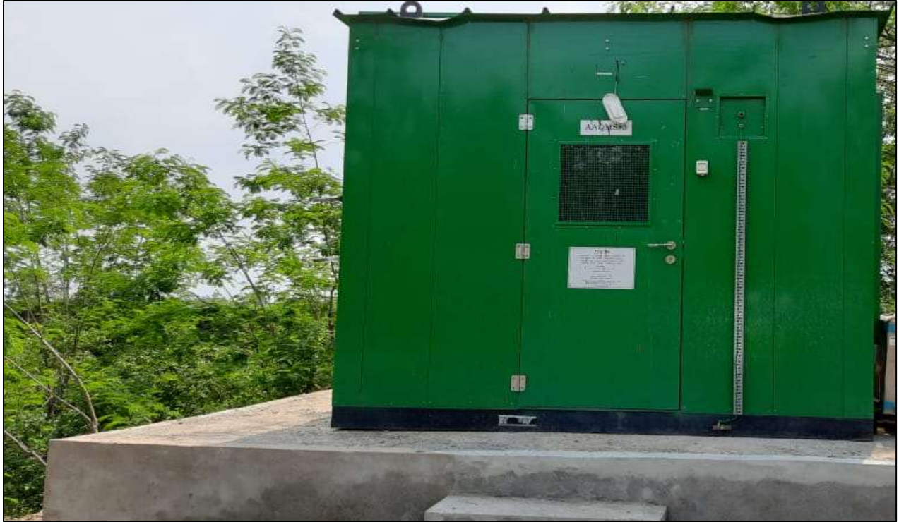
CAAQMS Installed at Crusher Area (Mines)
